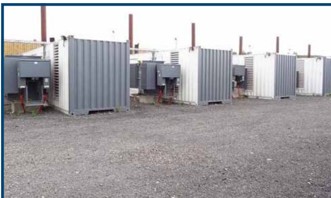
Diesel generators Photo: John Henderson at Environment Agency
