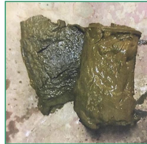
GSHP system - Biofilm chemically removed and 'captured' by the X-POT cartridge filter
