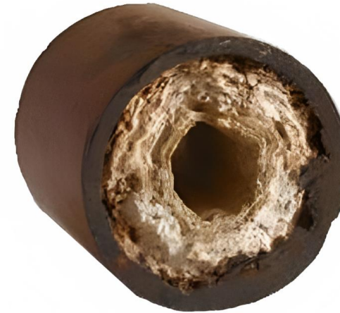
Pipework with heavy scale formation
