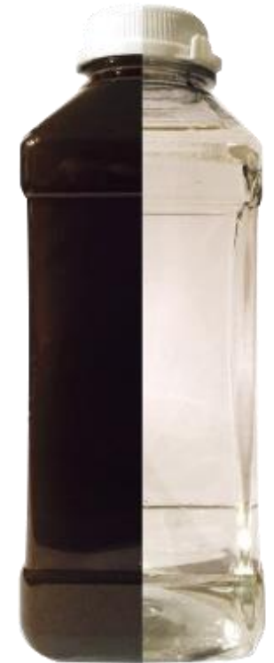
Sample from 2-year-old LTHW Heating System, before and after water treatment
