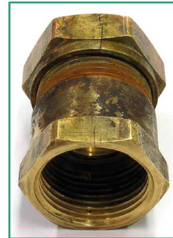
Stress corrosion cracking in brass fitting
