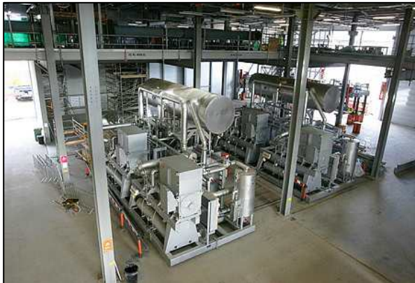
Two of the 4,6.6 MW chillers
