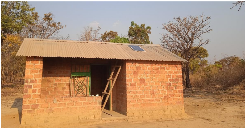
Figure 18:Installed solar panel
