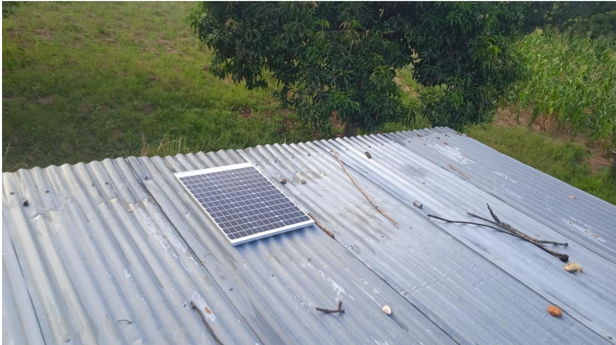
Figure 9 :Solar panel installed at a residential building in Zimbabwe
