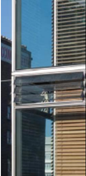
Figure 3.6 Active DSF Glass Louvre Opening
